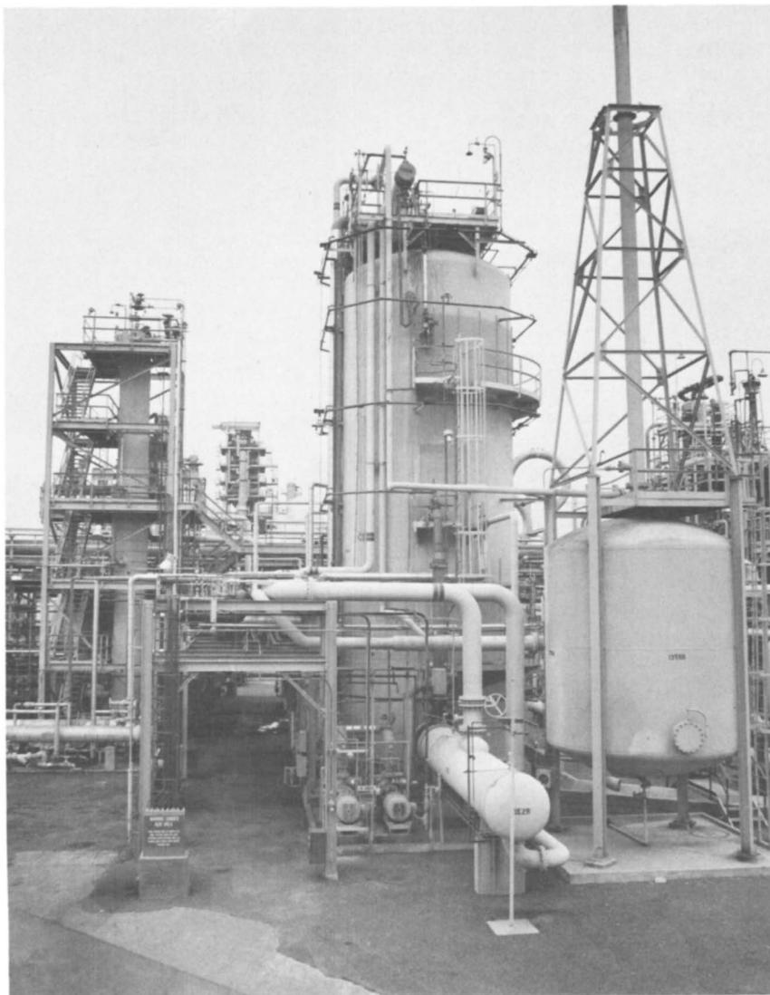
Figure 9. Single train alkylator used to produce 1.7 billion pounds of ethylbenzene per year
